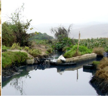
Figure 5: Blocked sewer, raw wastewater from the cities used for irrigation in agriculture. Source: H. Hoffmann
