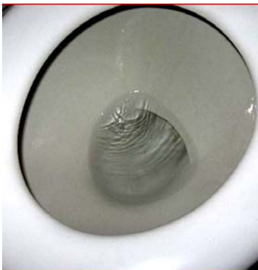
Figure 7: Water loss due to malfunctioning of water valves Source: H. Hoffmann
